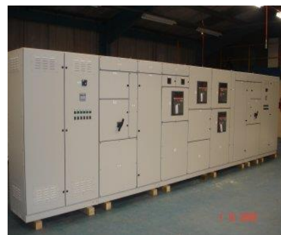
Multi-cubicle type assembly
