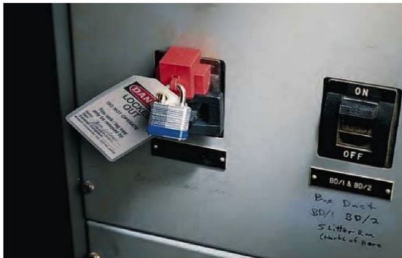
Main Breaker/Isolator Lockout
