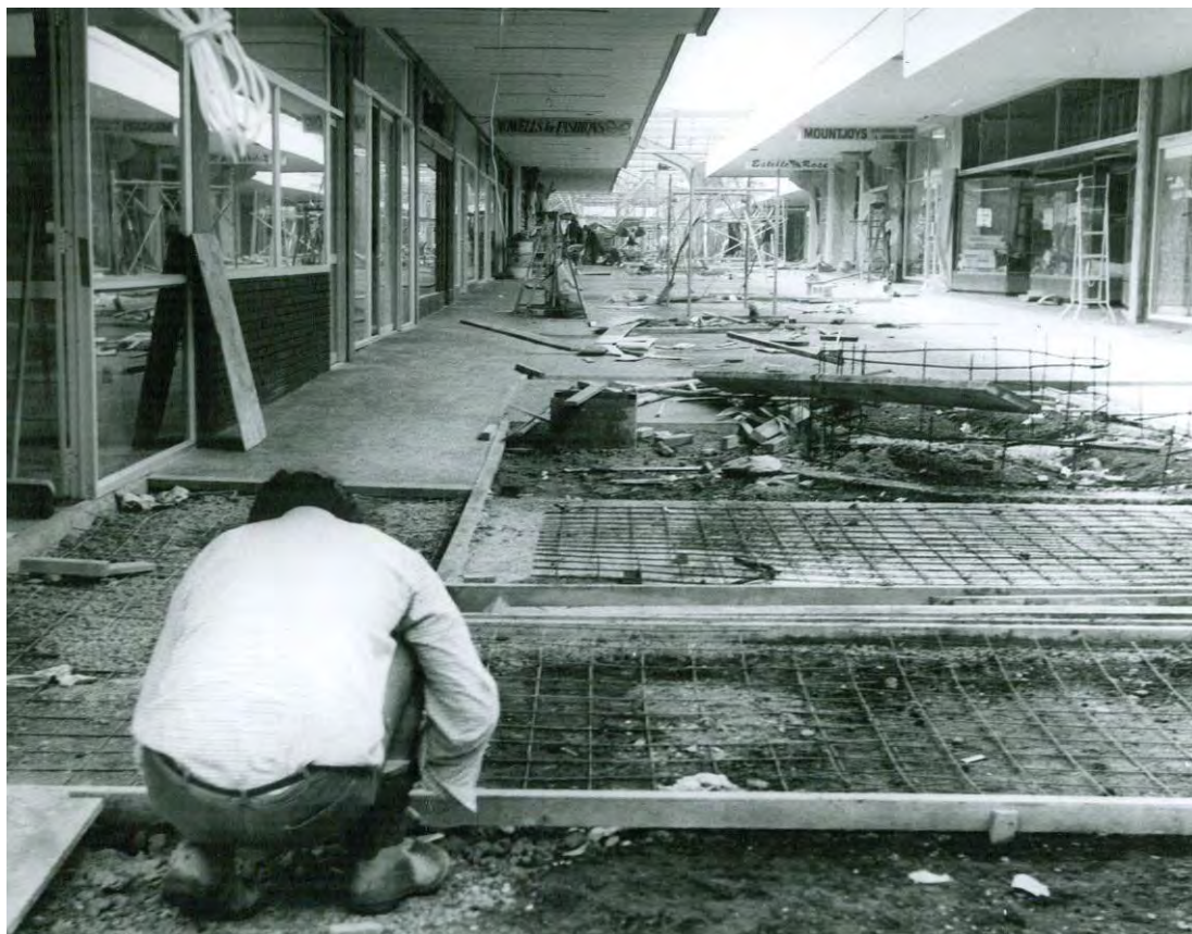
Figure 28: Work progressing on the Mangere town centre, with incomplete canopies in the distance. Source: South Auckland Courier Collection, Manukau City Libraries, 10 October 1971.
