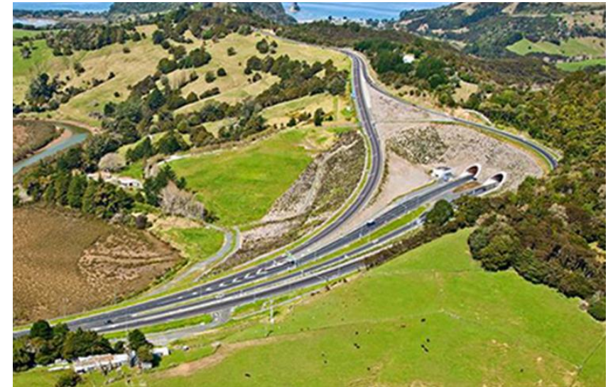
The first stage of the Ara Tūhono – Pūhoi to Wellsford Road of National Significance
